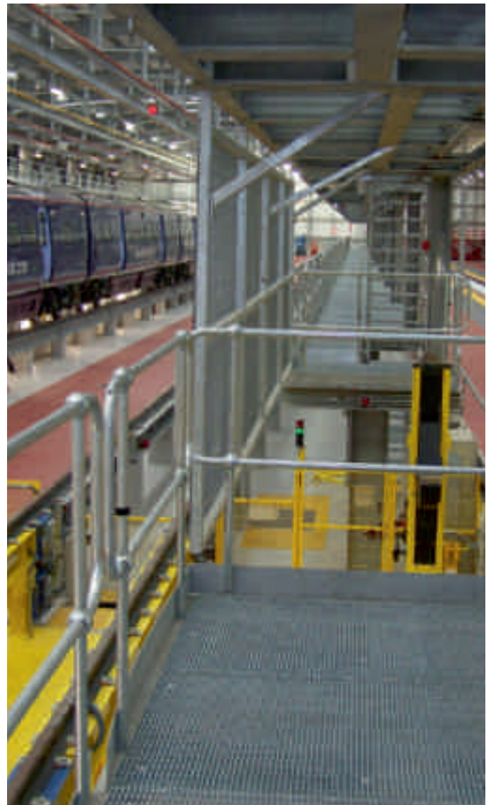
Access Design's rail project, utilising steel flooring, handrail, treads and galvanizing process.
